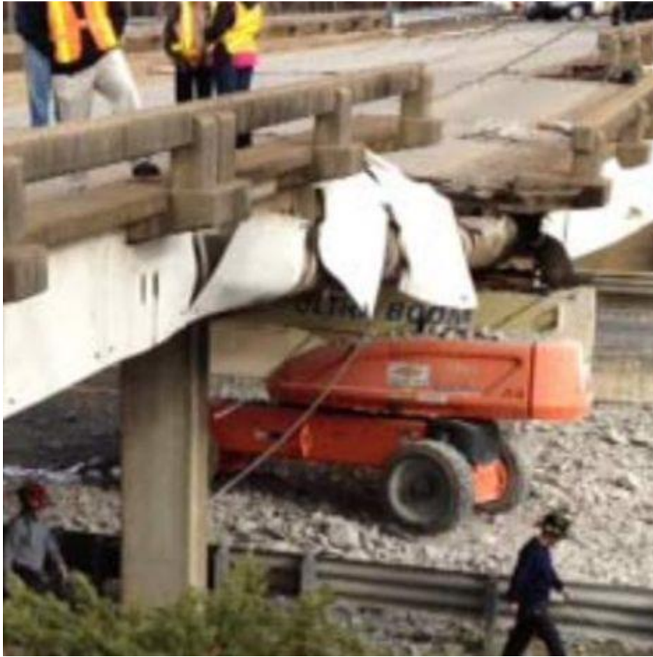
The bridge was damaged beyond repair
